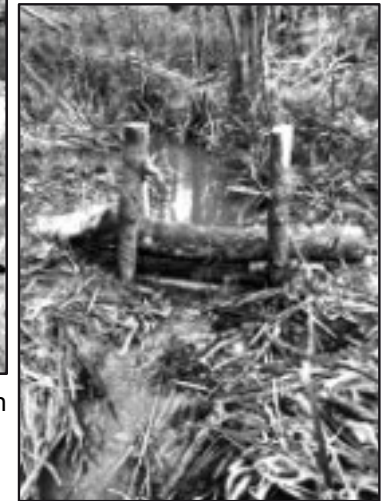
A leaky dam
