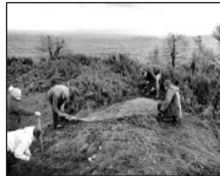
3: Measure chicken wire to size and peg chicken wire over the turf and sandbags so that they are held in place and can stabilise.
