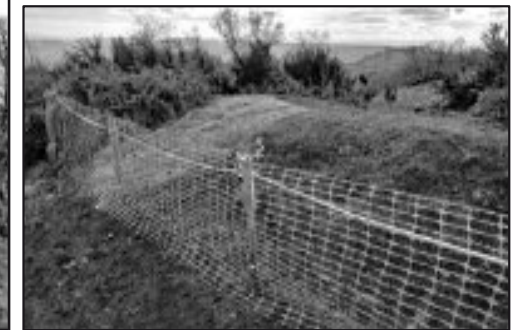
4: Put up fence to prevent people/livestock from getting on to the repair until it has bedded in.
