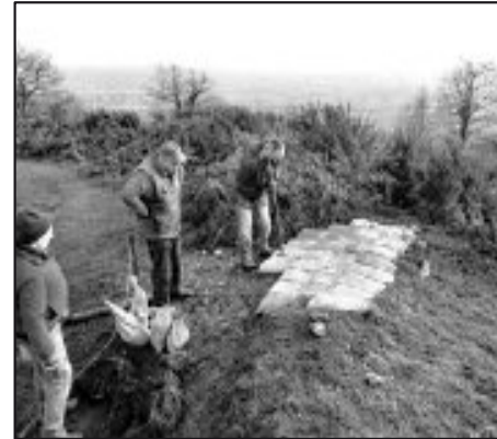
1: Fill sandbags and use the sandbags to fill in erosion scars, restoring the profile.
