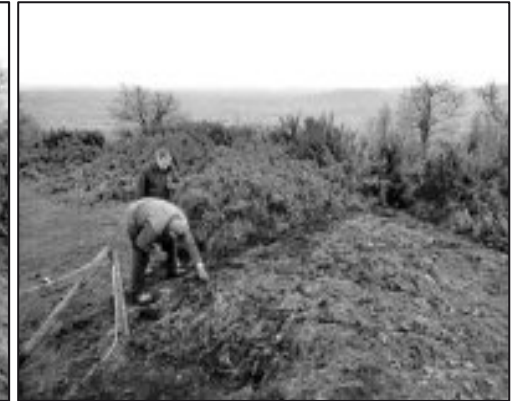
2: Cut turf from the rampart ditch. We used the ditch as it is the least botanically interesting. Lay turf over sandbags.
